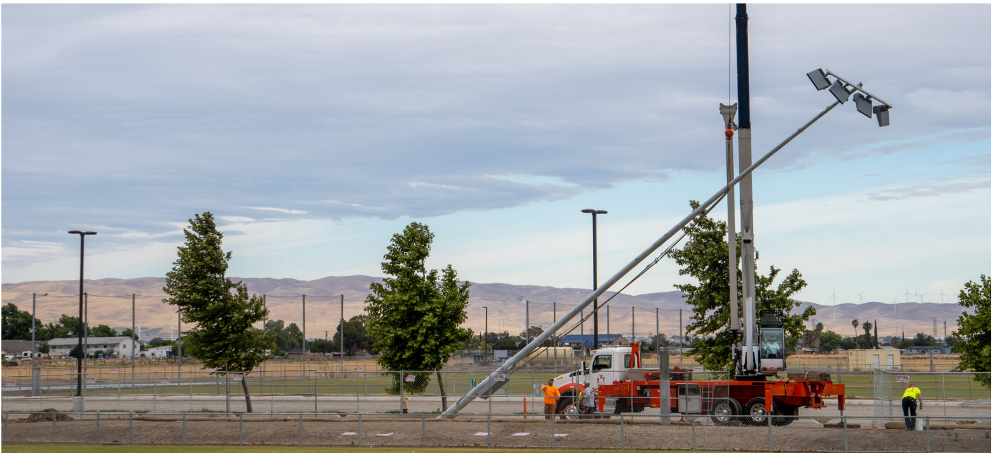
Phase 1 development of Legacy Fields Sports Complex has created new lighted fields for baseball and soccer.
