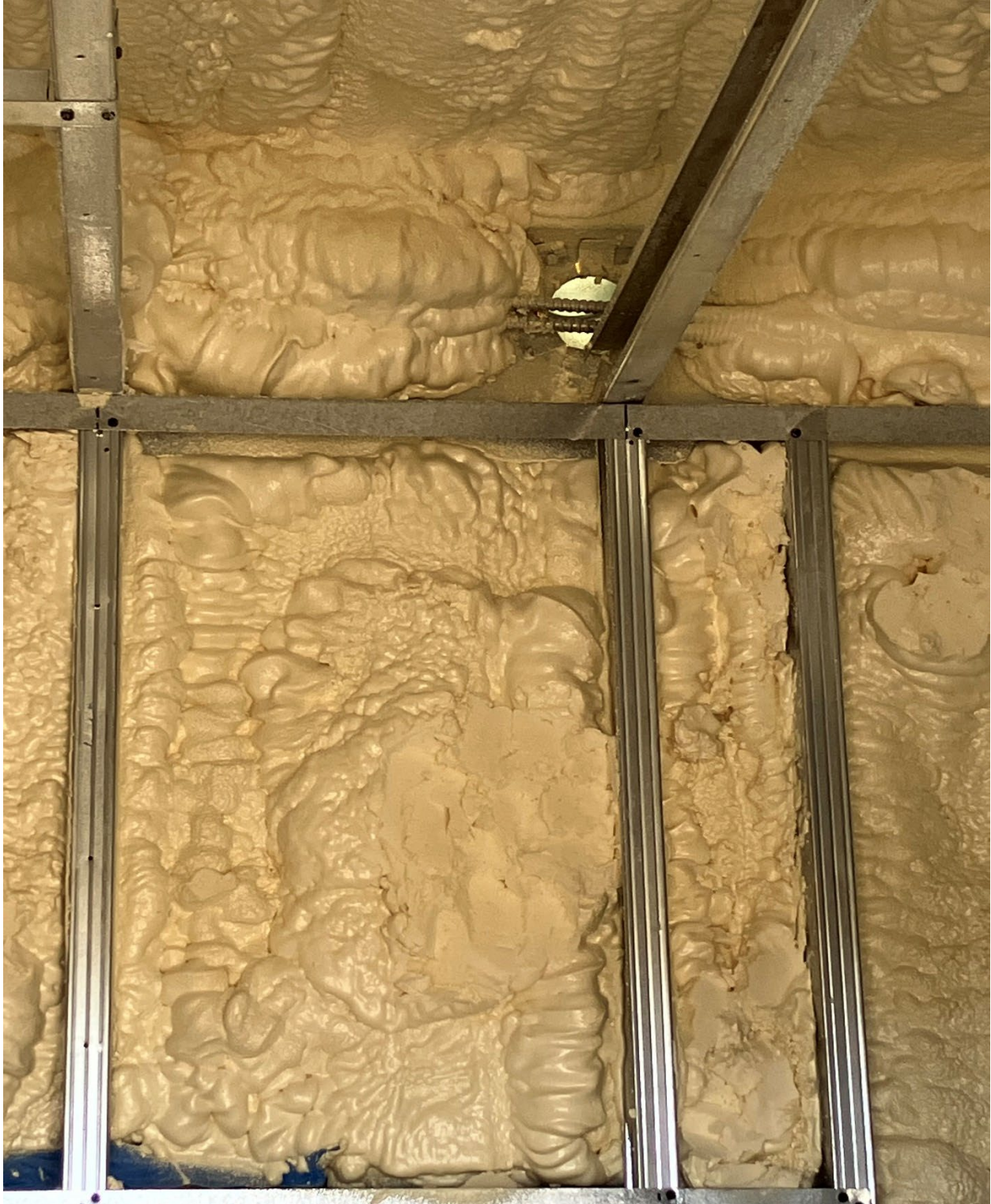
Figure 1 Photo 1: Port to external exhaust shows electrical wiring raceways conflicting with opening to allow duct from exhaust fans. This will be corrected.
