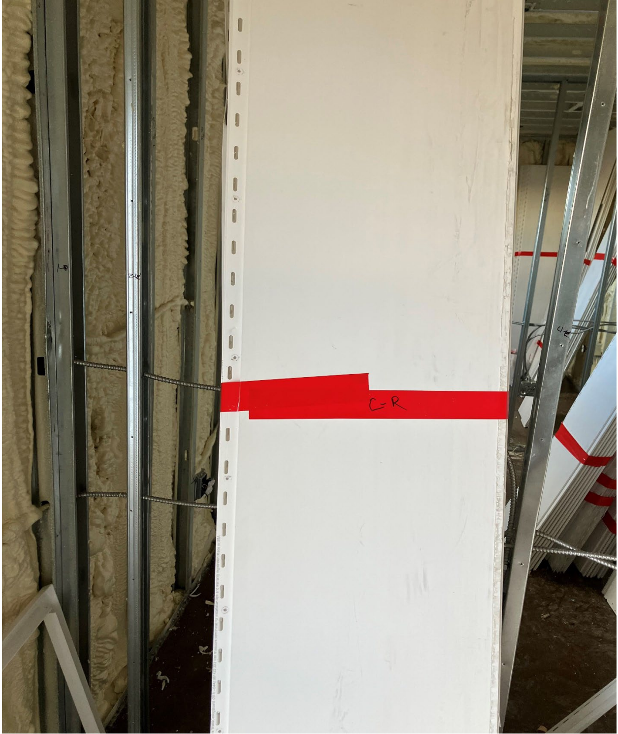
Figure 2 Photo 2: Shows paneling being labelled for removal for reinstallation upon completion of punch list items.
