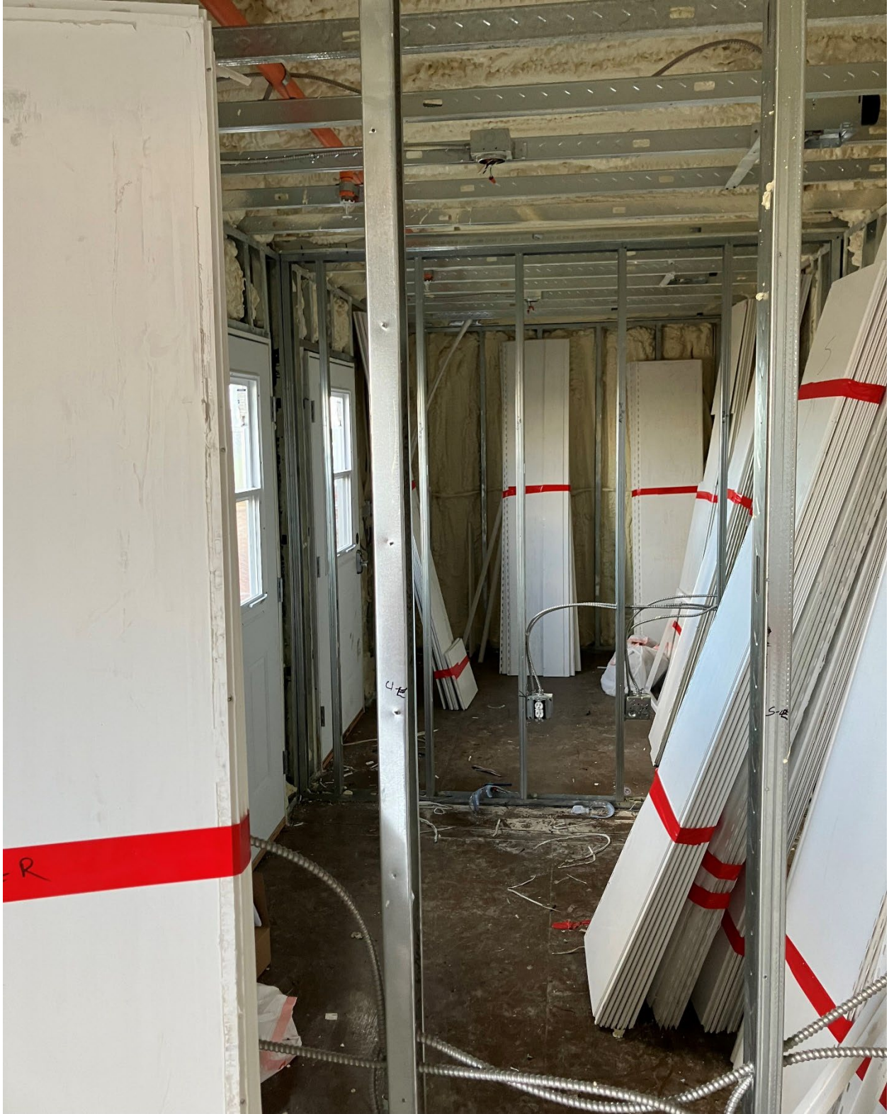
Figure ALL: These photos were taken March 3, 2023 of Modular unit M / 4 room configuration.
