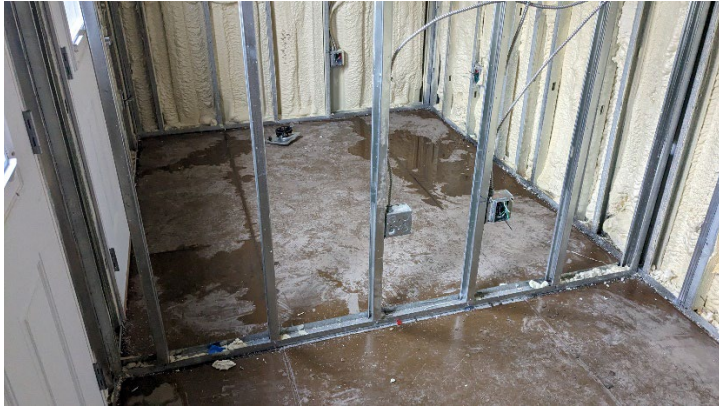
CC915 addressing water leaks with custom containers.
