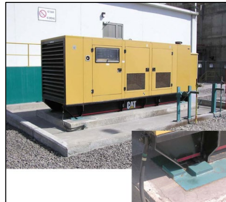
Figure 60 – Emergency Generator with Shear Lugs Added to Seismic Skid Mount
