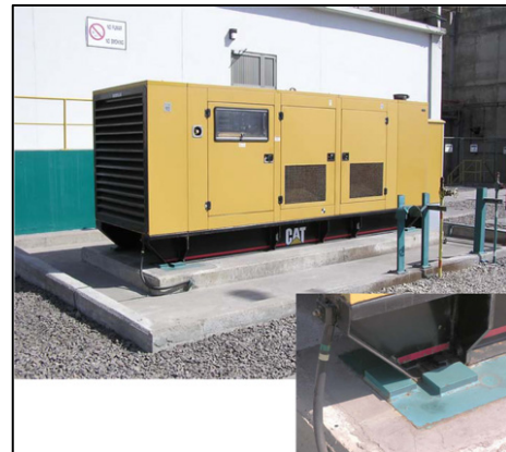
Figure 33 – Emergency Generator with Shear Lugs Added to Seismic Skid Mount
