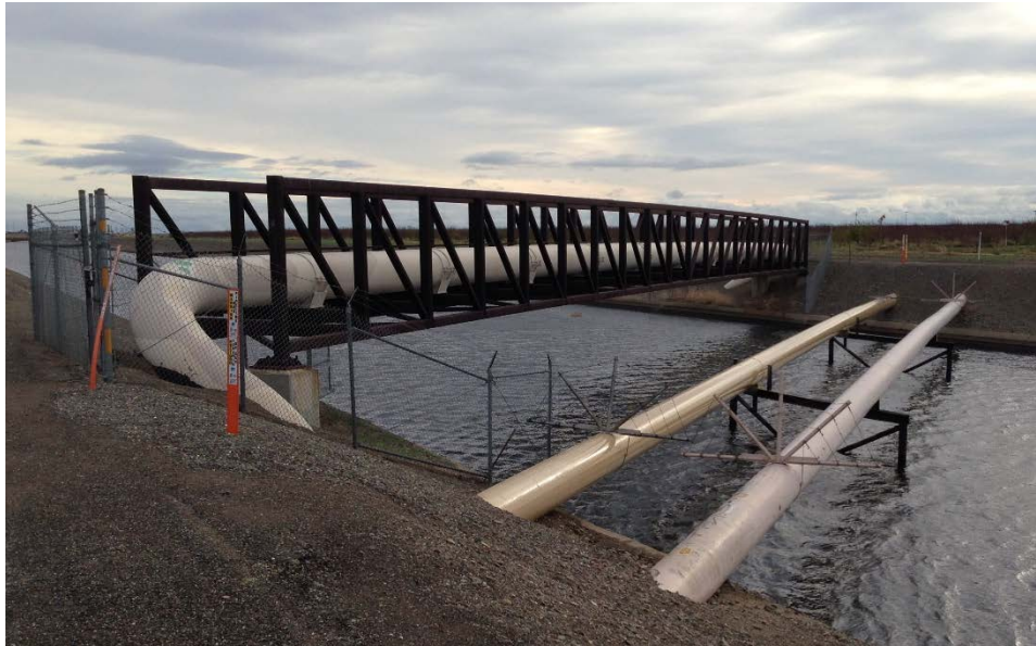
Photo 3. Taken from the east side of the Delta-Mendota Canal looking west, at canal mile 14.49. Shows a pipeline crossing.
